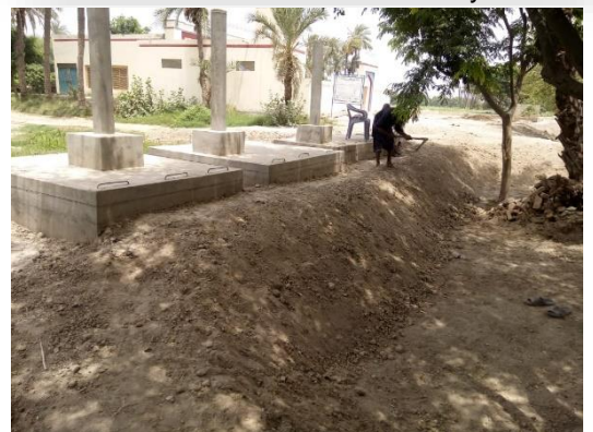
Sewerage Treatment Unit (STU)
